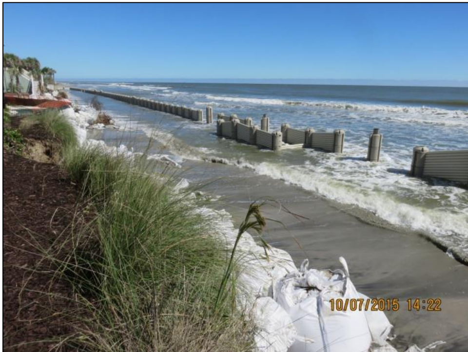
Figure 2-31. WDS at Beachwood East following Hurricane Joaquin; view towards the northeast (source: SCDHEC-OCRM)
