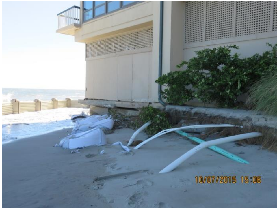
Figure 2-21. Erosion at Ocean Club building following Hurricane Joaquin (source: SCDHEC-OCRM)
