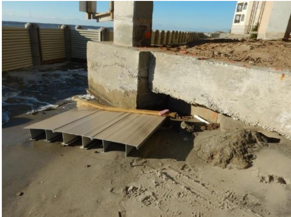
Figure 2-25. Dislodged vertical porous panels at Ocean Club on February 25, 2016 (source: SCDHEC-OCRM)
