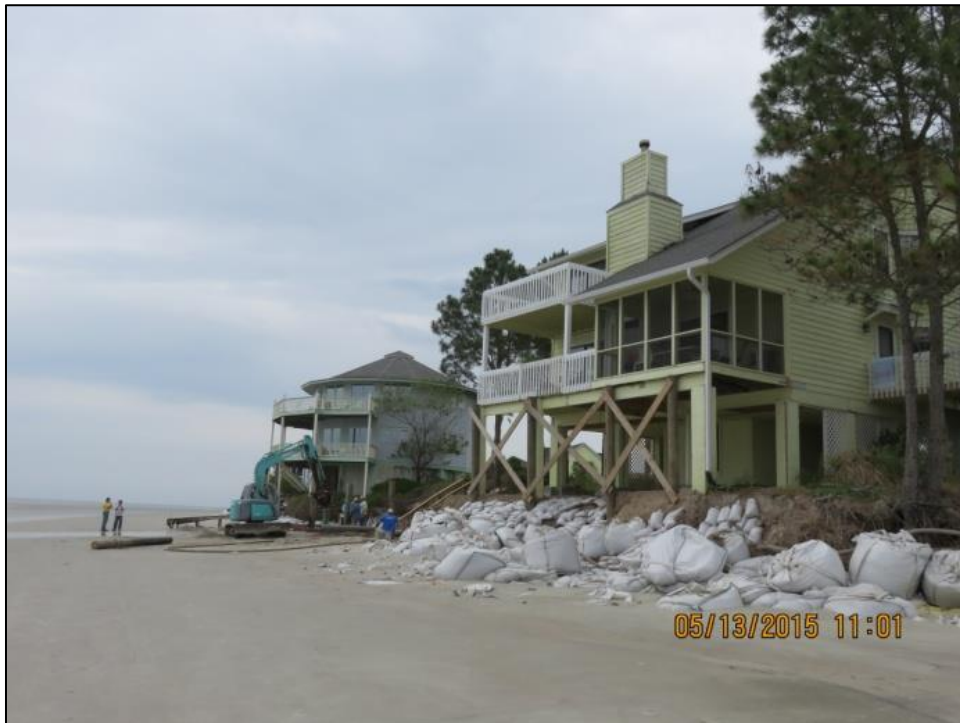
Figure 2-10. Shoreline conditions at lot 52 prior to WDS installation
