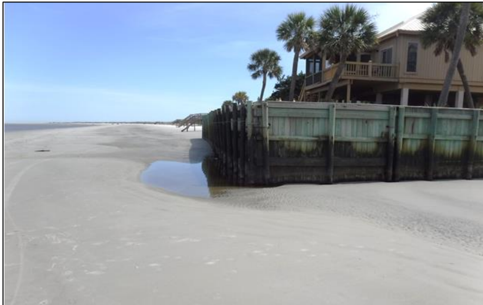
Figure 4-93. Scour at bulkhead on the beach (April 19, 2016)
