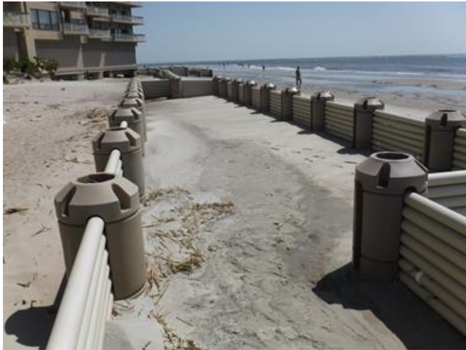
Figure 5-3. Low area between WDS tiers at Seascapes Villas (July 13, 2016)
