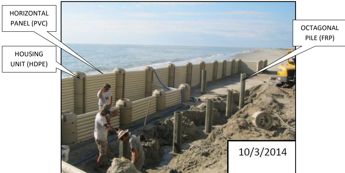
Figure 1-1. Photograph of WDS installation with annotation indicating WDS elements
