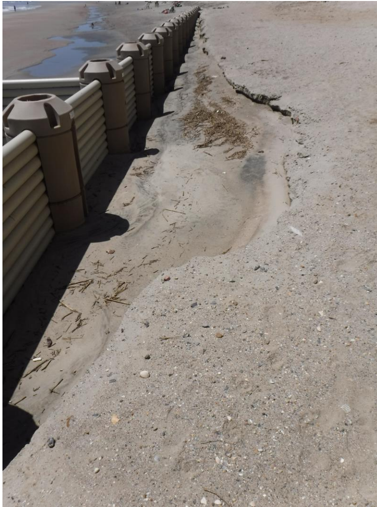
Figure 5-5. Erosion at Seascape Villas in area without scour beneath WDS (April 18, 2016)
