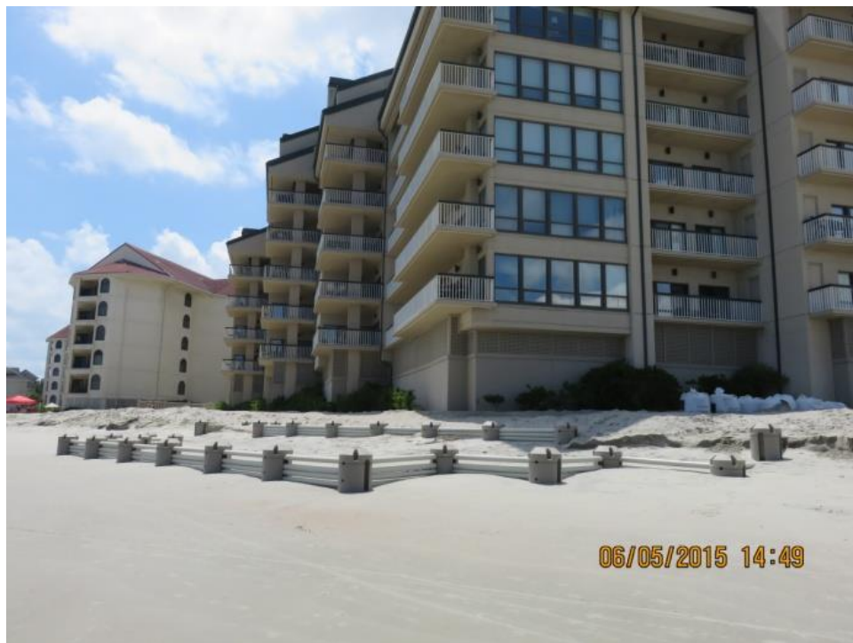
Figure 2-19. WDS at Ocean Club following June 2015 installation; view toward west (source: SCDHEC-OCRM)
