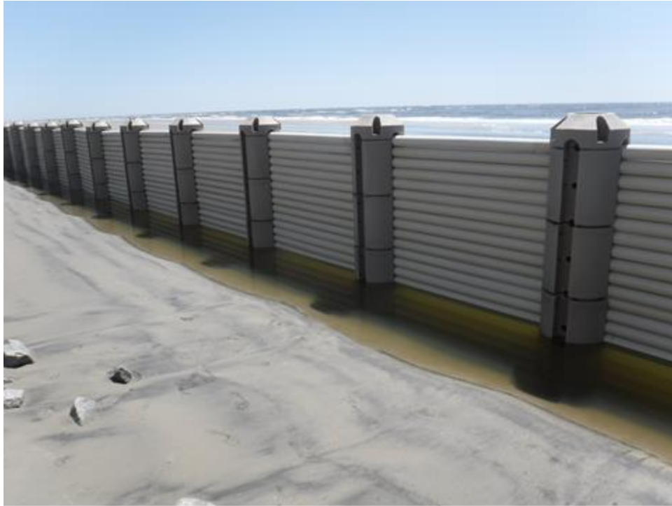
Figure 4-97. Scour at the BE WDS (April 18, 2016)
