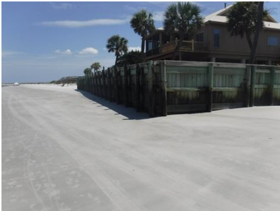
Figure 4-94. Scour at bulkhead on the beach (June 16, 2016)
