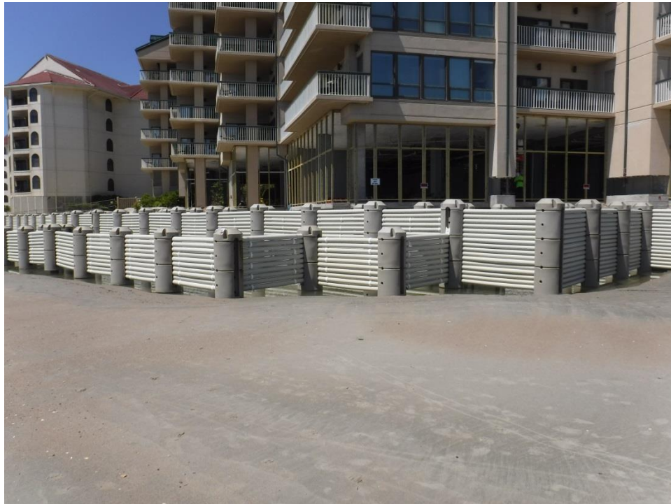
Figure 4-101. Scour at the OC WDS (April 18, 2016)
