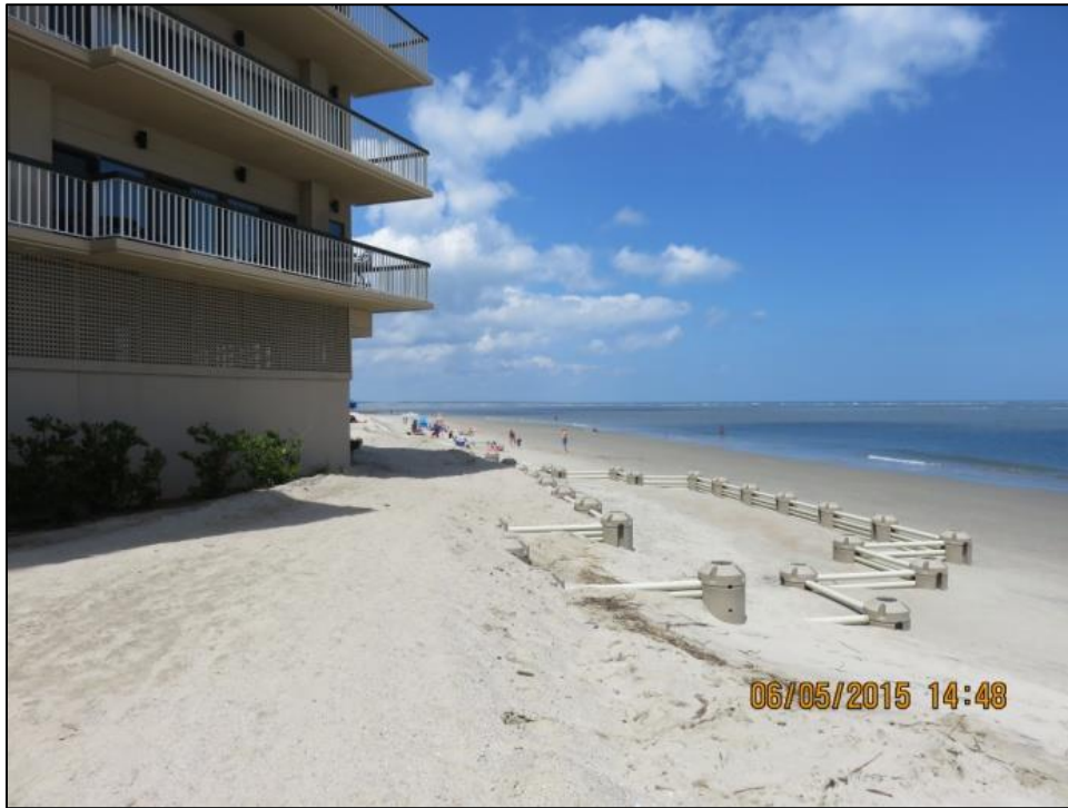
Figure 2-18. WDS at Ocean Club following June 2015 installation; view toward northeast (source: SCDHEC-OCRM)
