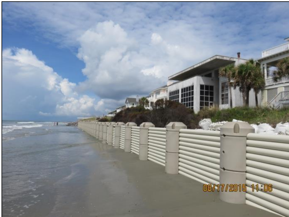
Figure 2-29. WDS at Beachwood East following August 2015 installation (source: SCDHEC-OCRM)
