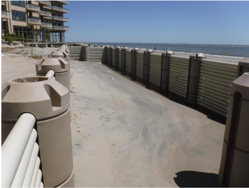
Figure 4-99. Scour at seaward tier of the SV WDS (April 18, 2016)
