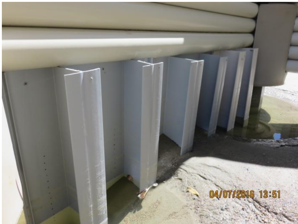
Figure 2-24. Vertical porous panels installed beneath horizontal WDS members at Ocean Club (source: SCDHEC-OCRM)
