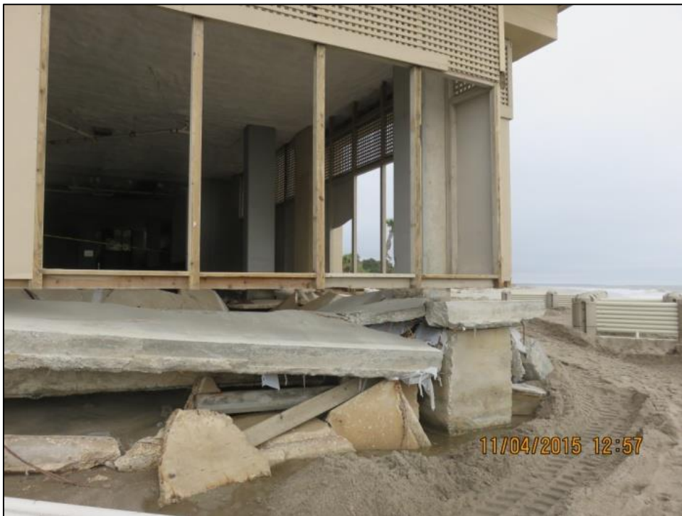
Figure 2-22. Undermining of Ocean Club building and collapse of slab in parking garage (source: SCDHEC-OCRM)
