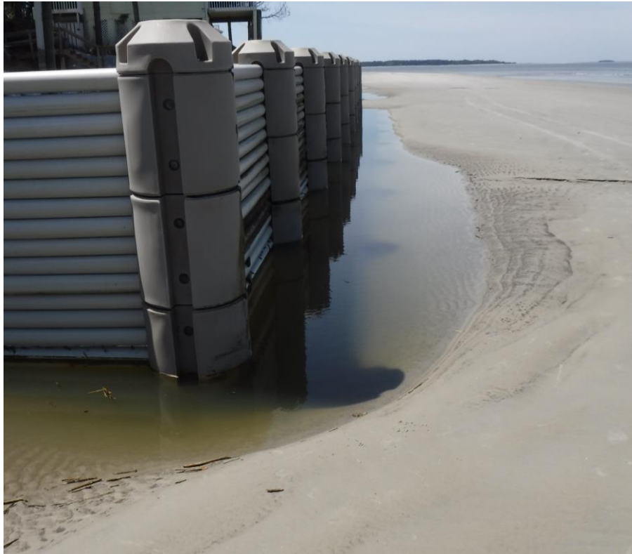
Figure 4-95. Scour at the Harbor Island WDS (April 19, 2016)
