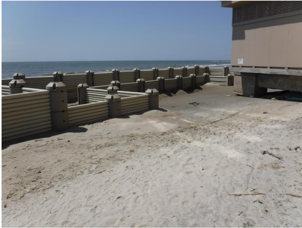
Figure 4-77. July 13 photograph from east side of OC looking south
